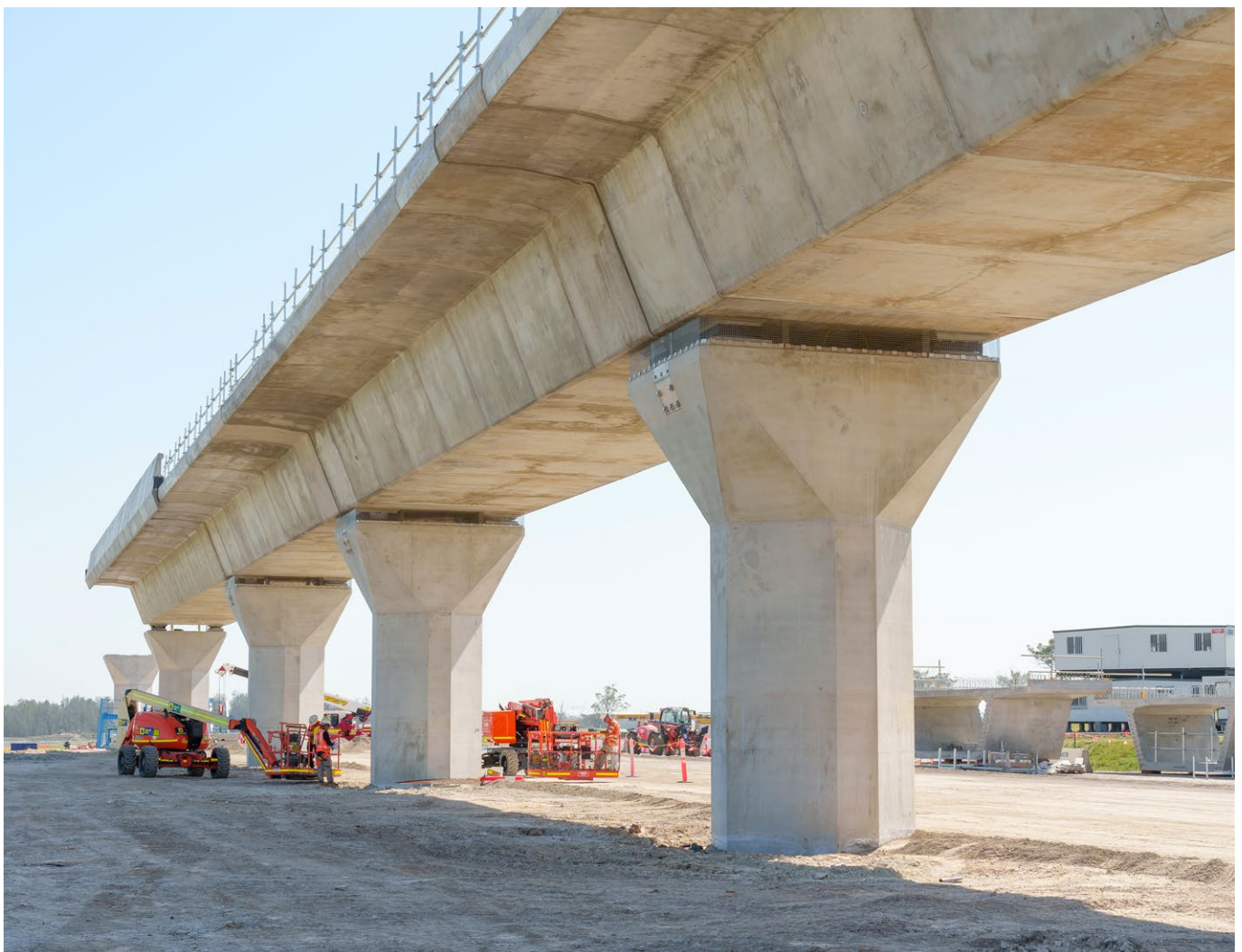
■ Sydney Metro – Western Sydney Airport viaduct construction, Copyright State of NSW (Transport for NSW)
