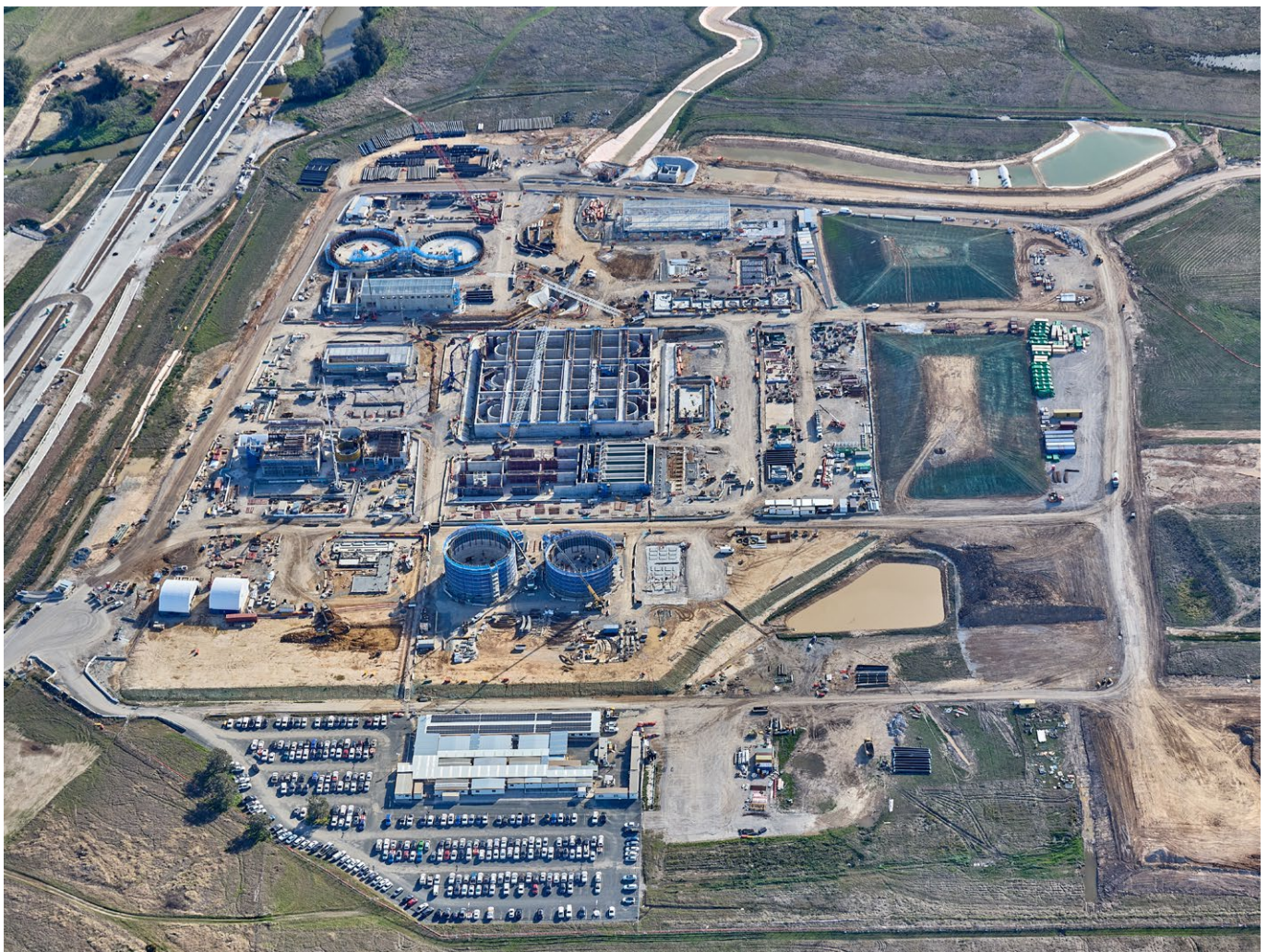
Upper South Creek Advanced Water Recycling Centre (AWRC) under construction, Sydney Water
