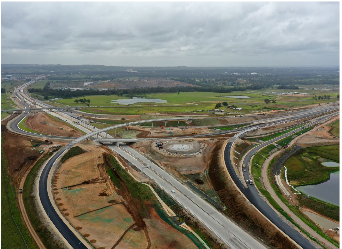
| Sydney Metro – Western Sydney Airport, M12 Motorway, Elizabeth Drive and WSI Airport under construction, Transport for NSW
